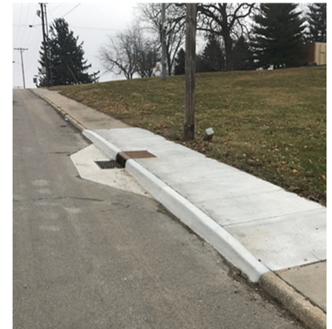
Figure 6: Photo displaying a sidewalk with no vegetated barrier. The sidewalk is directly against the roadway with nothing in between.
